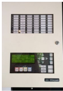
Fire Panel in SVO (Located SVO 1 st Floor near Weisz House Doors & at 2 nd Floor Nursing Station)
