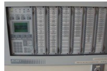
Fire Panel in SVTOO (Located SVTOO Main entrance, each nursing station and 3 rd Floor across from elevator)
